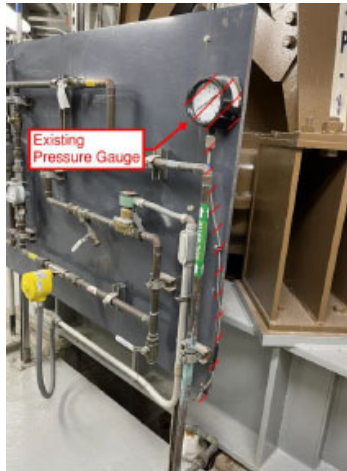
Pumps 1-5 Manual Suction Gauges
