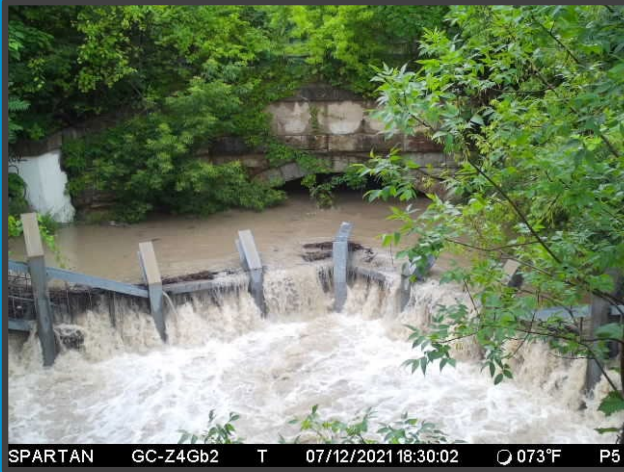
Airport Debris Rack
