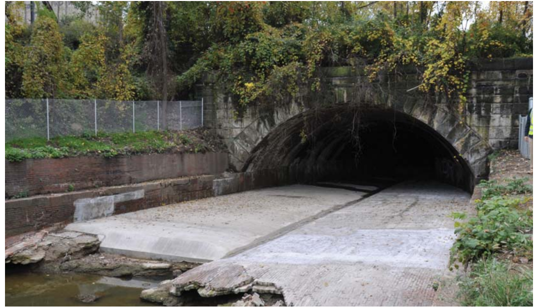
Photo of Walworth Run CSO 080 discharge outlet into Cuyahoga River
