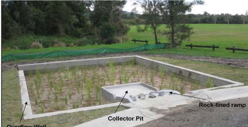
Small infiltration basin with sediment collector pit and vegetation
