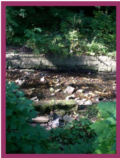
Leaning Wall with Undermined Base ◀
