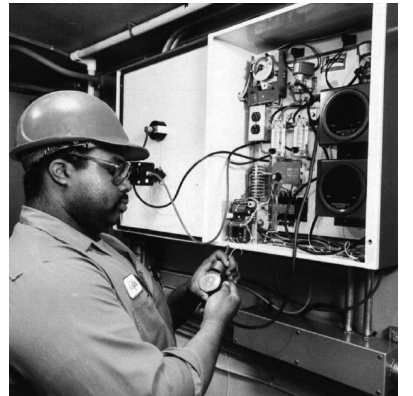
The CSO control system's network of programmable controllers, flow level sensors, and computer-controlled mechanical gates prevent wastewater from spilling into area waters.
