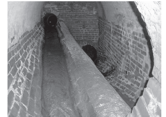
A combined sewer under East 107th Street. During heavy rains, a combination of rainwater and diluted untreated wastewater flows over the weir to an outfall.
